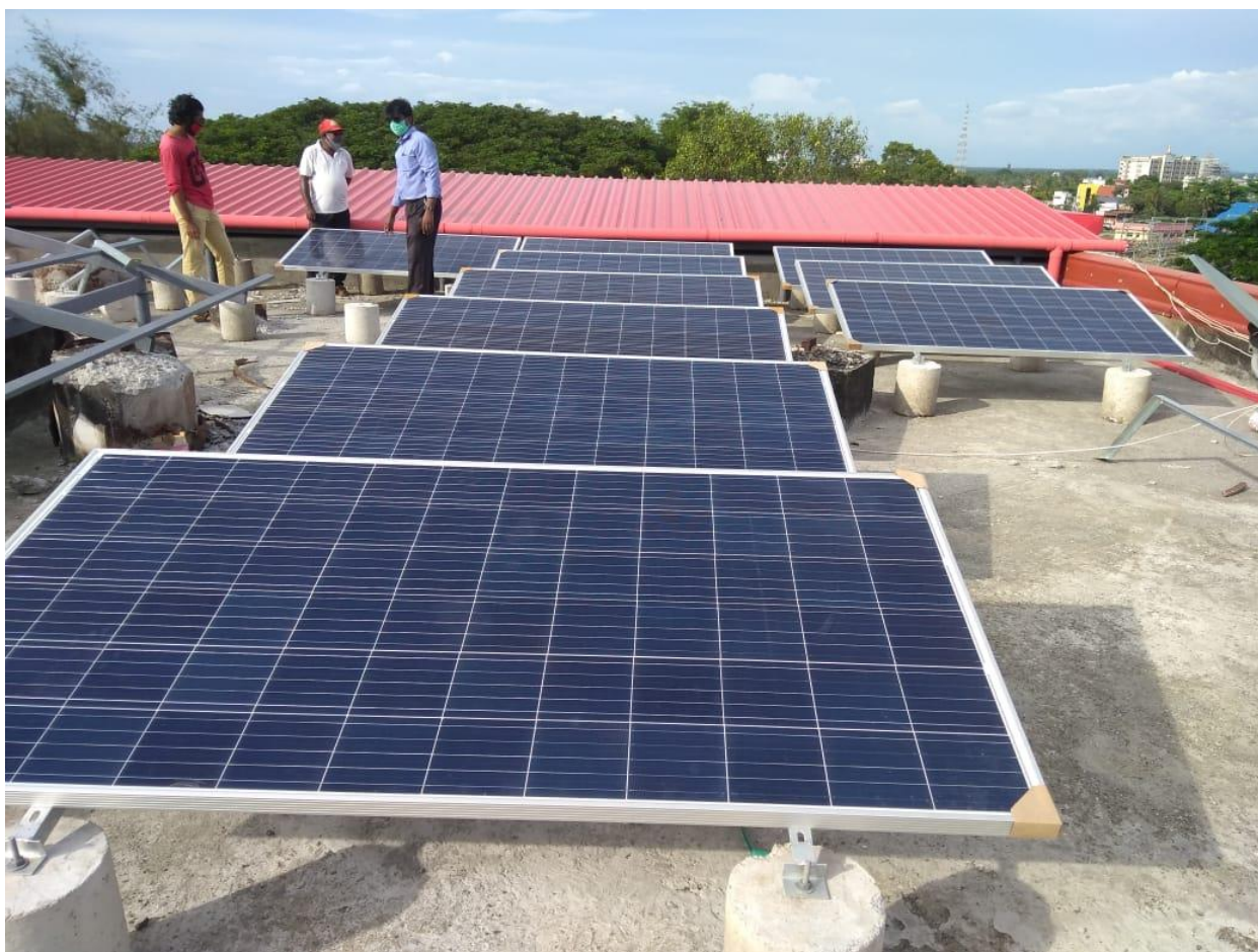
Figure 7.1 Solar Modules, 325W/330Wp Multi crystalline (TATA )
